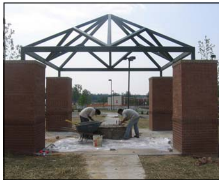
The Leisure Landscapes crew is shown installing the lighting and completing the stonework for the statue pedestal for the Pavilion.
